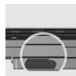
DMX power supply units inside the body of the luminaire
